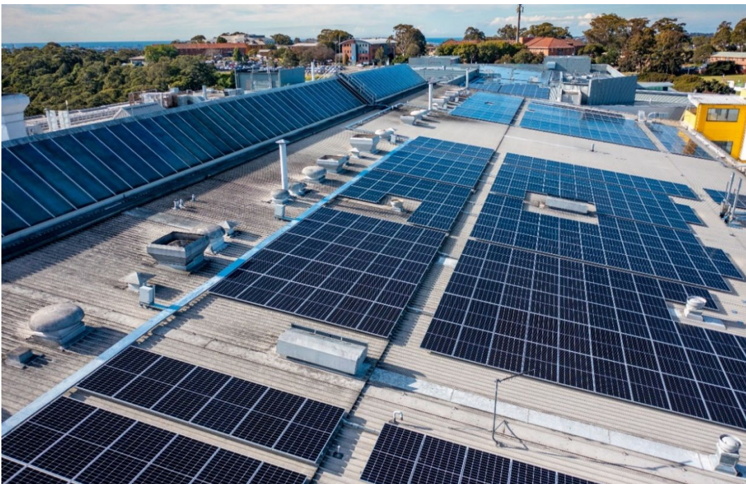
Agencies can help alleviate pressure on the electricity grid during high demand periods. Photo: rooftop solar panels, John Hunter Hospital, Newcastle. Credit: ©NSW Health
